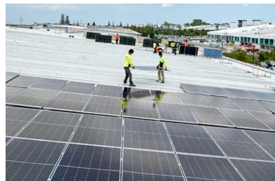
ROOFTOP SOLAR PANELS BEING INSTALLED AT OUR EAST TĀMAKI, NEW ZEALAND CAMPUS IN THE 2026 FINANCIAL YEAR.
